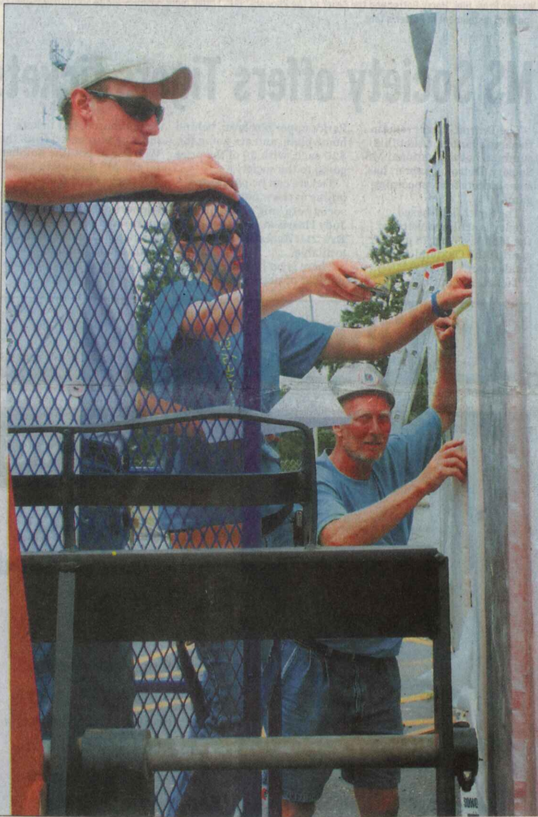
Students Larry Bukowski (left) and Sonia Tereszczenko install insulation on a house that will represent Lawrence Technological University in the National Solar Decathlon Competition in Washington, D.C. Working with them is Jeffrey Kruse of the Michigan Regional Council of Carpenters and Millwrights.
