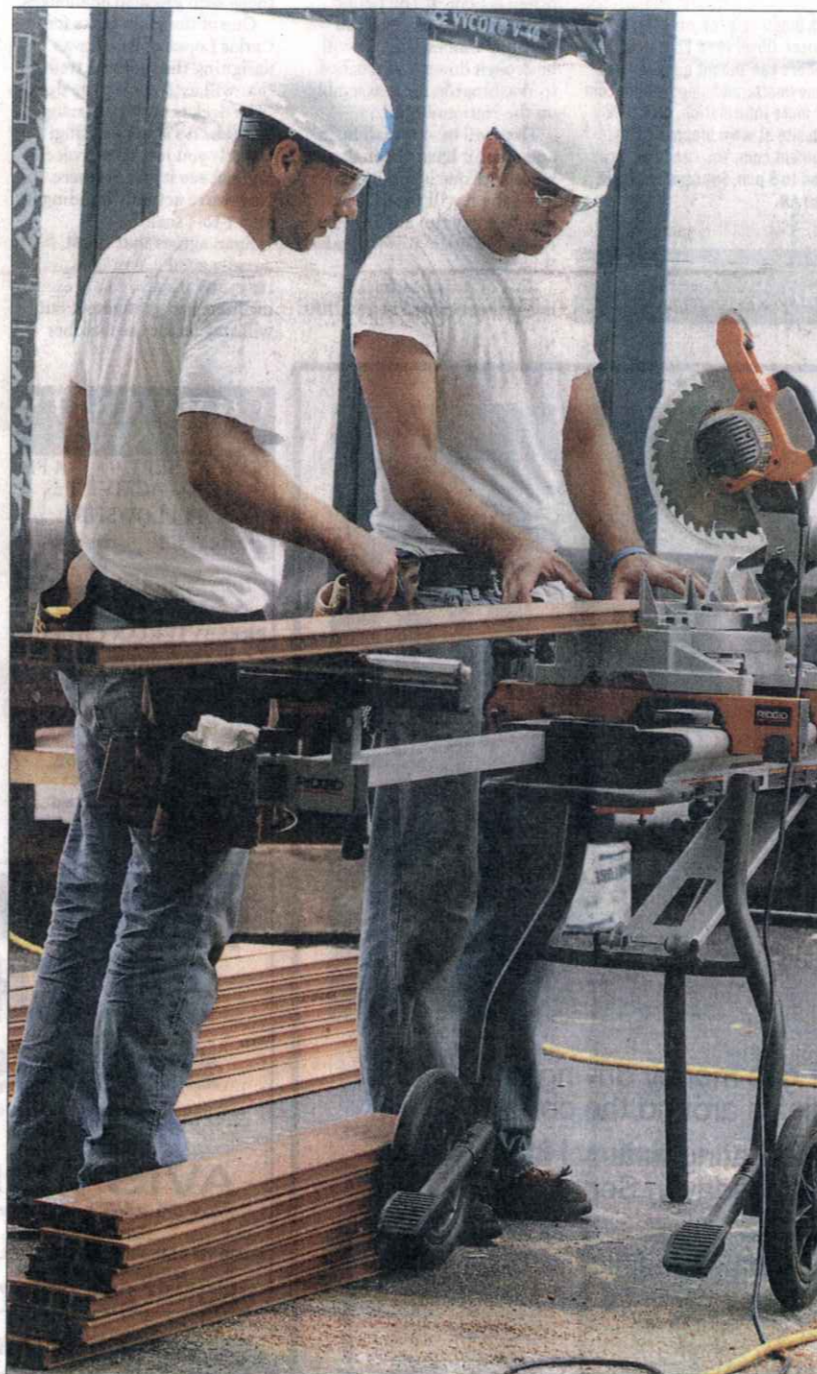
Carlos Lopez (foreground) of Brazil and Scott Salvaggio of Sterling Heights, both members of the Lawrence Technological University solar house architectural and design team, work on the composite deck of the home.
