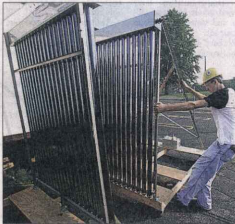
Tominac inspects tubes that will be used to heat water in the solar house being built for a national competition.
